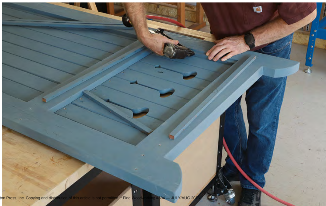
Front stops. Hartman pin nails front stops around the sides and top of the panels to help hold them in place. To avoid trapping water, he doesn't place a stop at the bottom.
