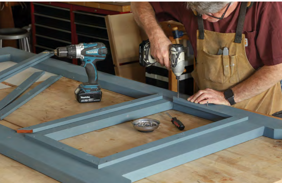
Back stops. After painting the frame and the panel slats, Hartman screws back stops around both openings in the gate frame. He'll screw the slats to the stops.
